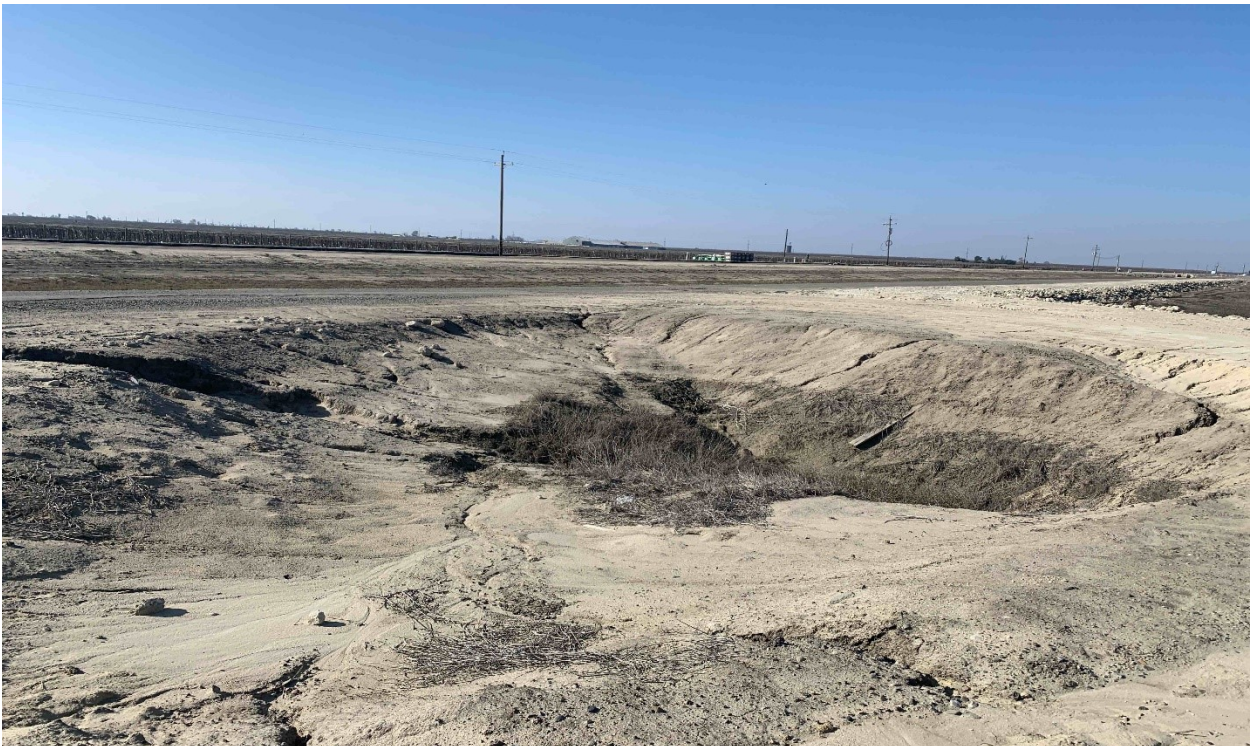
Photograph 4. View of sedimented culvert at southeastern corner of the project site, facing southwest.
