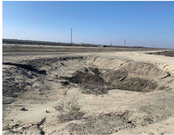
Photograph 4. View of sedimented culvert at southeastern corner of the project site, facing southwest.
